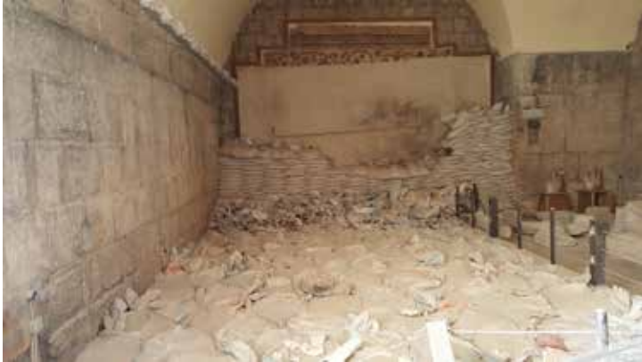
Interior of the Ma'arra Mosaic Museum, located in Northwest Syria, showing the results of a barrel-bomb of June of 2015.
