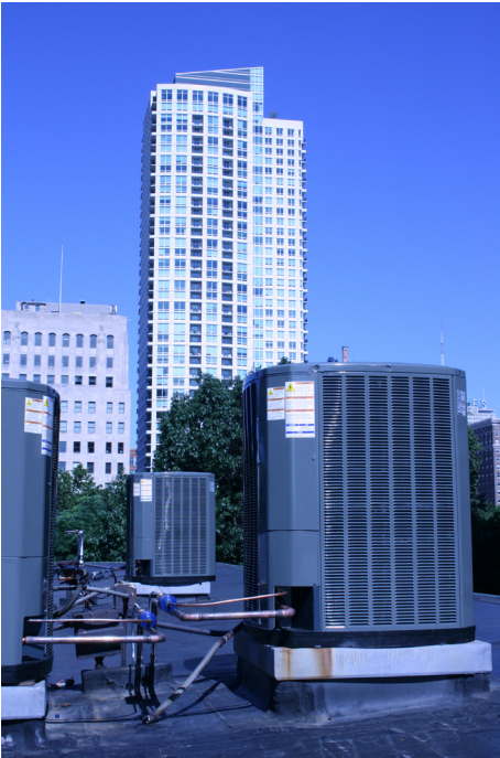
New air conditioner condenser units installed on Athenaeum roof.
